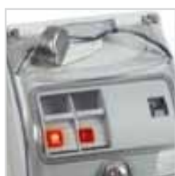
Failed fuse warning light
